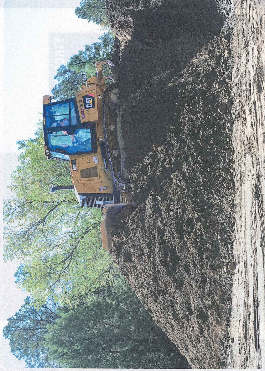
Lead remediation is expensive. A bulldozer moves the last pile of dirt with high lead content at the former Prescott Sportsmen's Club Shooting Range, April 18, 2017 in Prescott, Arizona. Cleanup costs approached $1.6 million. (Photo courtesy Les Stukenberg at The Daily Courier)
